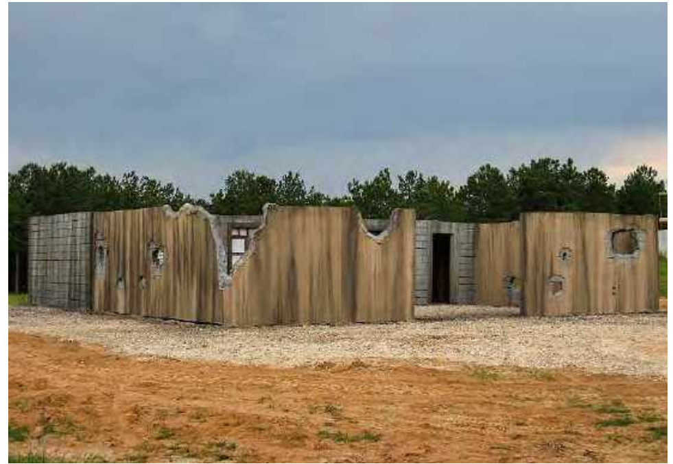
Damaged Mud Courtyard Wall
