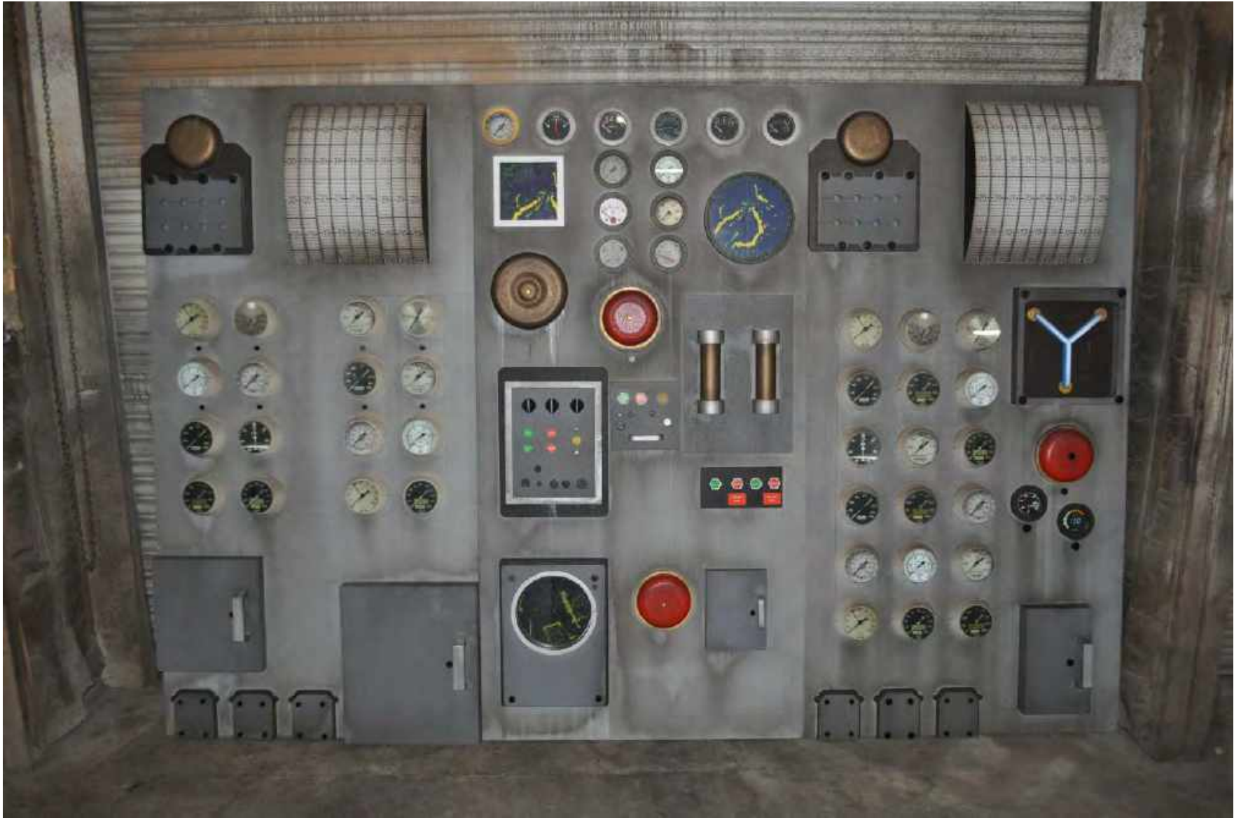
Ship Control Room
