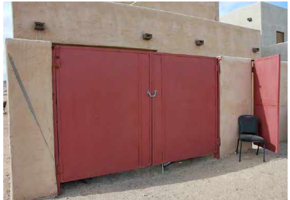
Metal Vehicle and Personnel Gates
