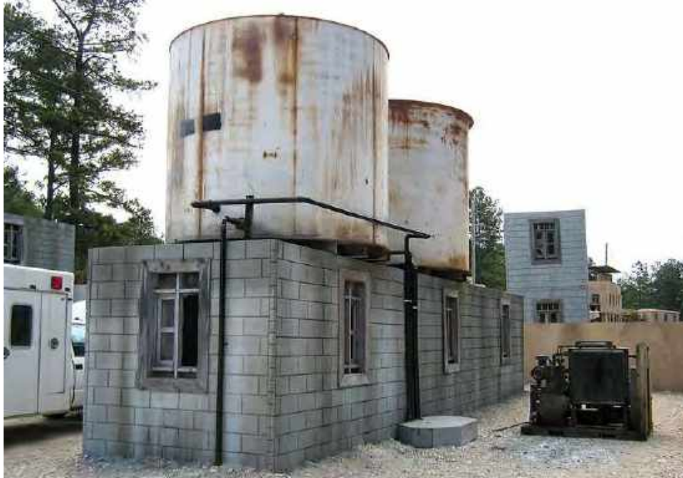
Industrial Pump Station
